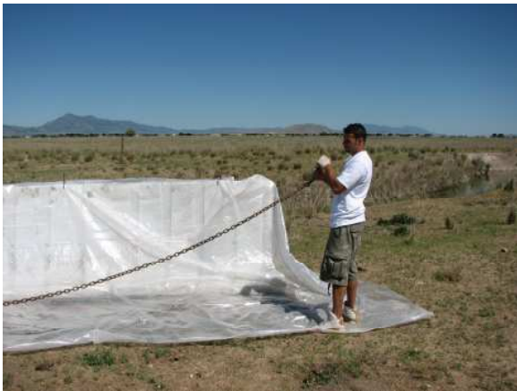
(Step 7 A) Alternative method to trenching is to use 3/8 inch chain to keep plastic in place.
